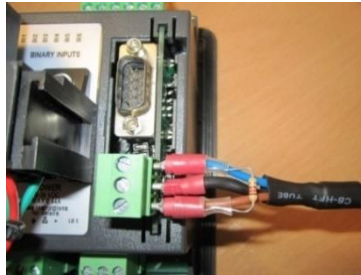
MAIN SCO 10 communication wire end
