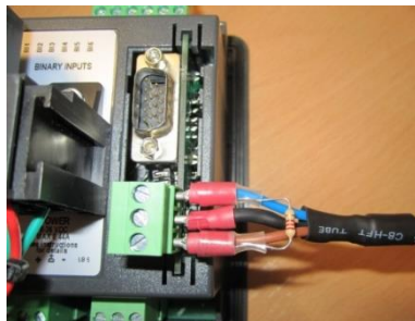
MAIN SCO 10 communication wire end
